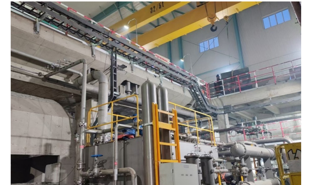
Reconstruction and Expansion Project of Power Generation from Sulfuric Acid Production and Waste Heat
